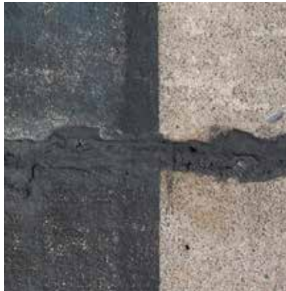
Even the expansion joint material has not been destroyed
