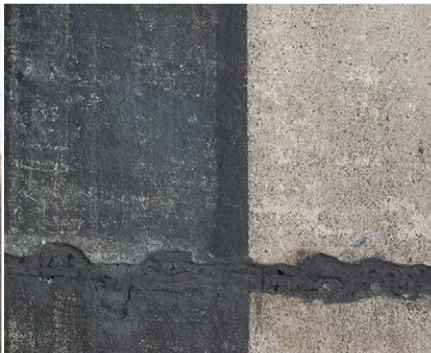
Even the expansion joint material has not been destroyed
